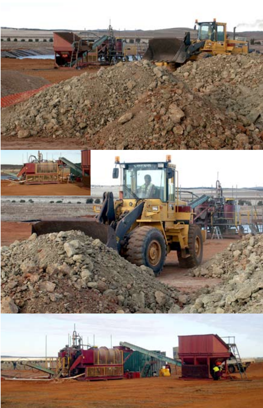
Figure 3 Kimberlite stockpiles and the DMS plant at the treatment site.
