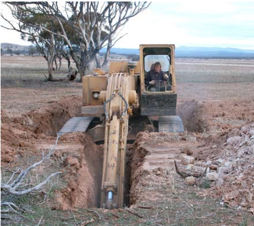
Figure 7 Excavator "benching down" to reach a depth of seven metres at the Franklyn Target.
